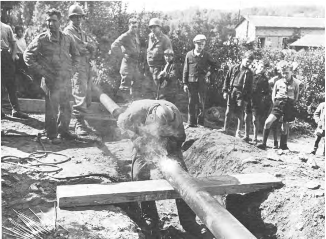
WELDING A SECTION OF THE POL LINE as it is extended eastward across France.
